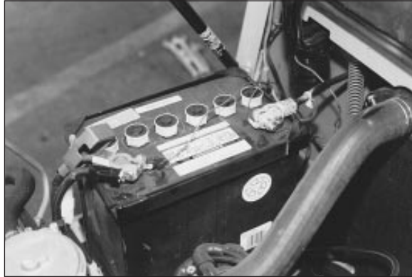
Figure 7: Connections to the lift truck battery.
